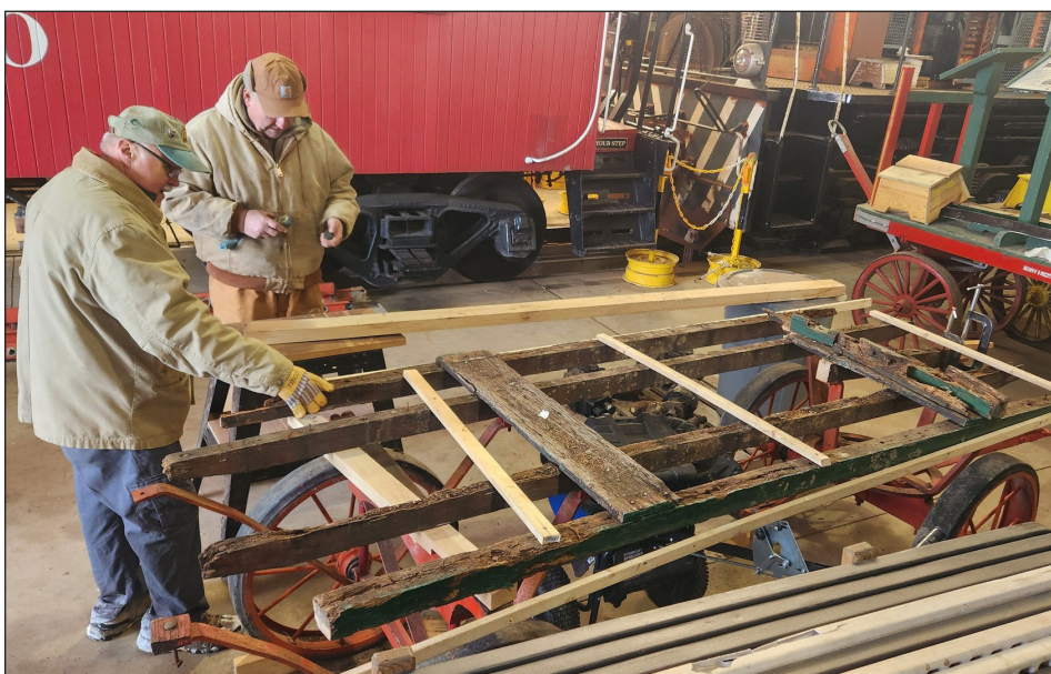
BELOW LEFT: Ernie Cole and Charlie Marks have one of our baggage carts stripped down to the frame for repairs and refurbishing. Charlie's son Jesse rebuilt the cart more than 20 years ago for a Boy Scout community service project!
